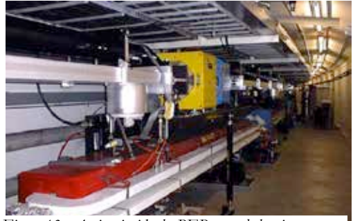
Figure 13: A view inside the PEP tunnel showing two rings stacked on top of each other for the PEP-II asymmetric B Factory.
