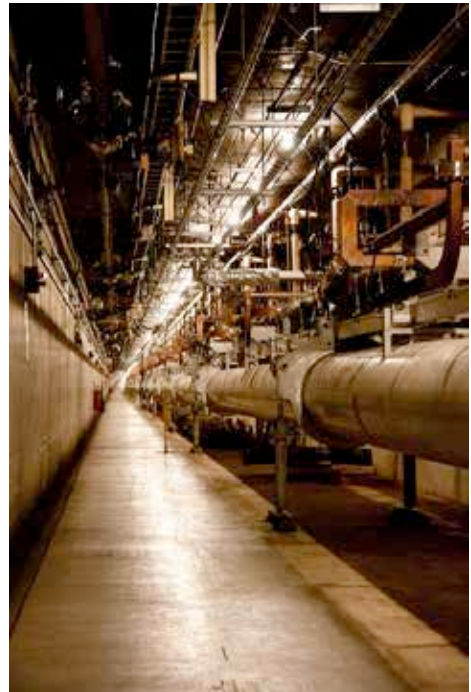
Figure 4: A view inside the two-mile SLAC accelerator tunnel showing the linac mounted above the alignment light pipe.
