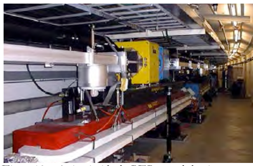
Figure 13: A view inside the PEP tunnel showing two rings stacked on top of each other for the PEP-II asymmetric B Factory.
