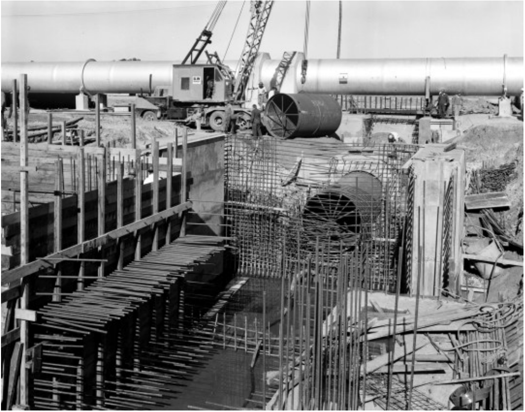
Figure 9: Warragamba Dam under construction. The photo shows No. 2 Cross Connection. Looking south at the cross pipe showing Mk. 26 under the crane. Partly constructed 84 inch valve chamber in foreground.
