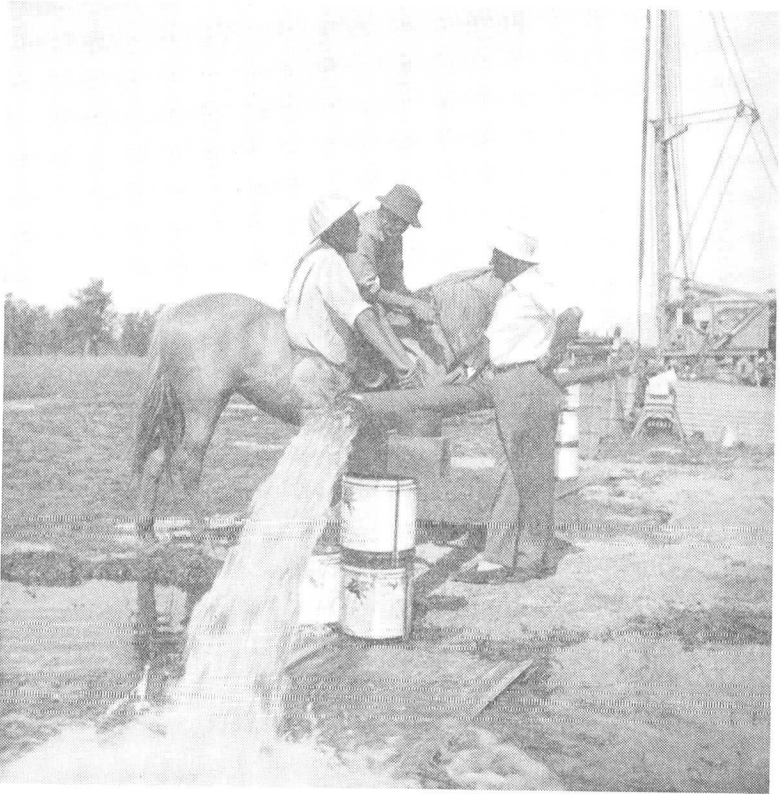
Ten-inch diameter bore, 350 ft. deep, located in Lachlan Valley, being tested at 40,000 g.p.h. The bore could yield 100,000 g.p.h. Constructed by Water Conservation and Irrigation Commission. (See page 97.)
