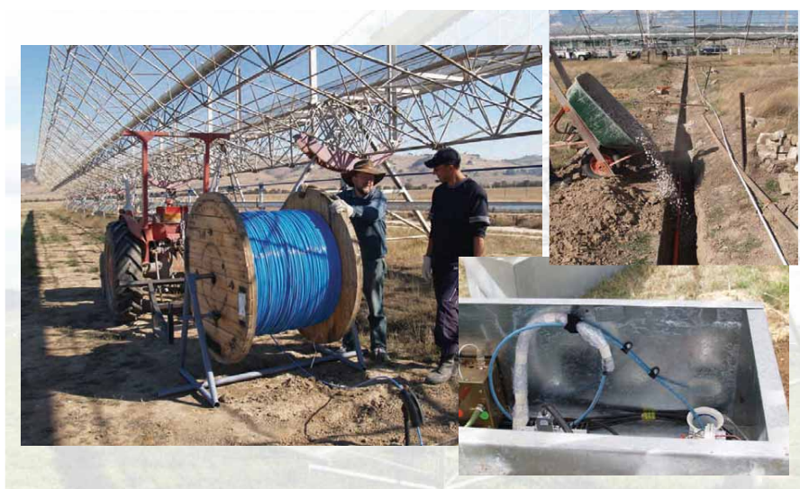
Fibre optic cables being laid as part of the upgrade to the Square Kilometre Array Molonglo Prototype
